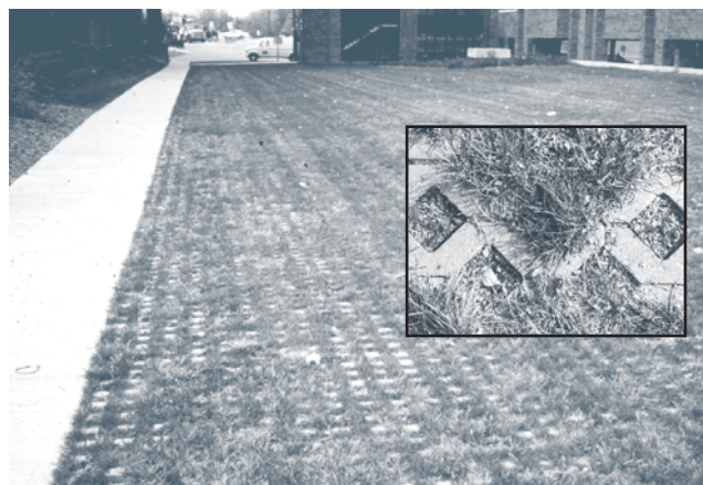
The DuPage County government complex uses permeable paving techniques for an emergency access road.
