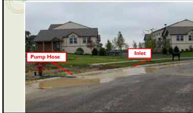
De-Watering Illicit Discharge
